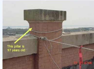
Anchor point for lifeline rope not evaluated prior to use
