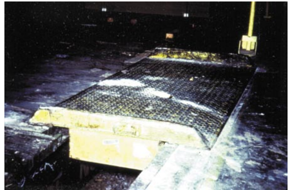
A projection below the surface prevents the dock board from shifting off its support.
