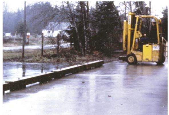
A bull rail at an unused edge of a dock reduces the risk of a forklift wheel slipping off.
