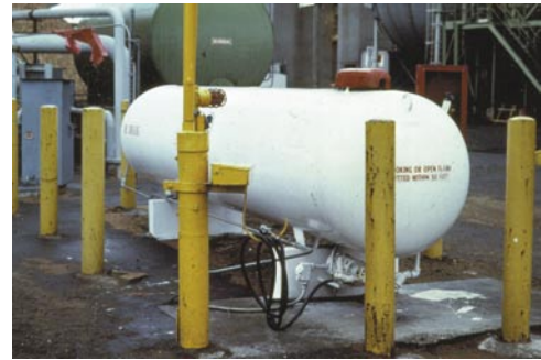
Propane tank used to refill the forklift LPG tank is protected against vehicle damage by heavy posts.
