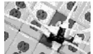
Overloads are a major cause of fires.
