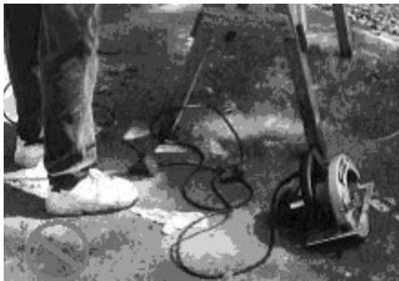
Combinations of hazards increase risk.
